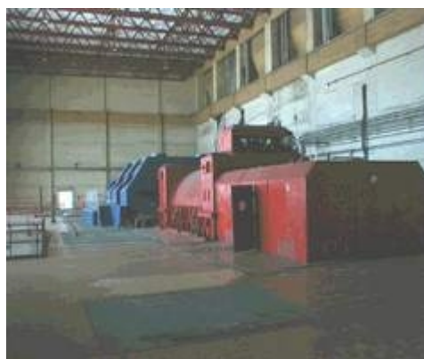
The interior of the generator
